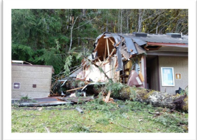
Before: Damage resulting from deferred maintenance at Loon Lake Recreation Area.
