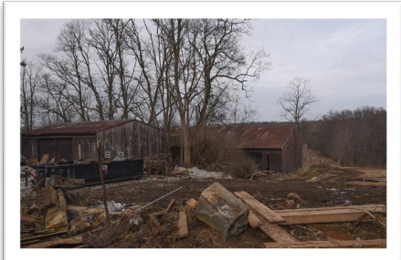
Before: Vacant structures at Cuyahoga Valley National Park created public hazards and hindered reforestation efforts.
